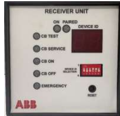
Receiver Unit - Mounted in LV box of the panel
